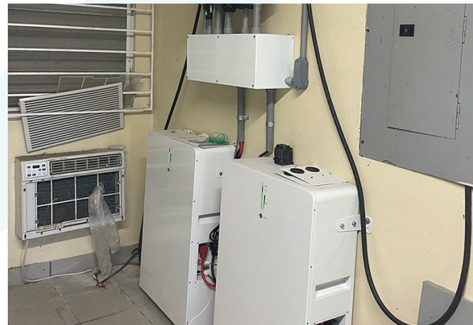
Picture 4. Solar System Batteries
