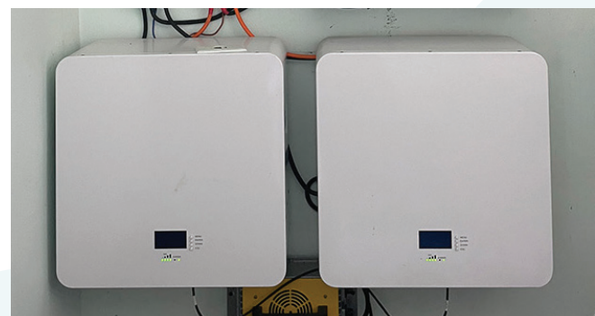
Picture 11. Solar System Batteries
