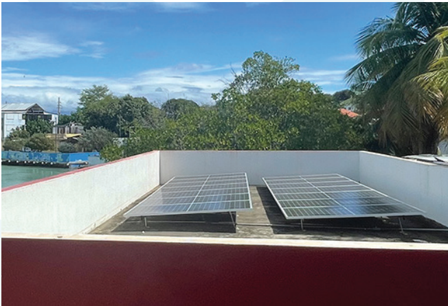
Picture 40. Solar Panels
