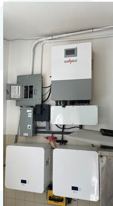
Picture 35. Solar System Batteries
